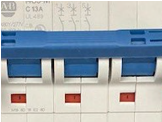
Bank 1 Breaker Closed/Hot
