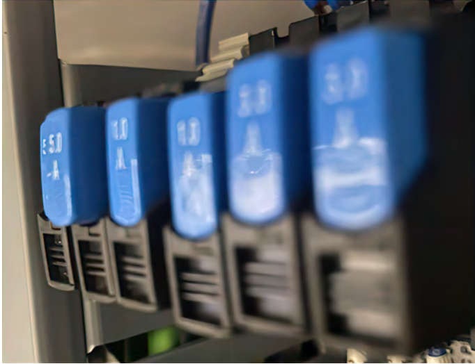
Bank 3 Breaker Tripped
