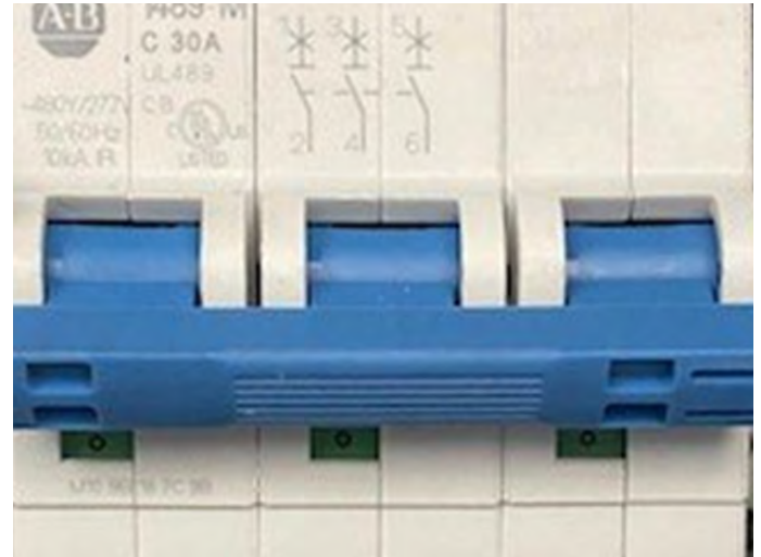
Bank 1 Breaker Open/Tripped
