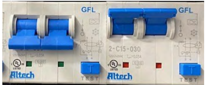
Bank 3 Breaker Open/ Tripped (OFF)
