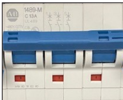
Bank 1 Breaker Closed/Hot
