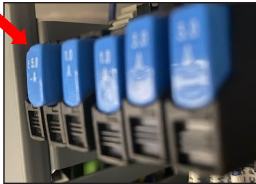
Bank 3 Breaker Tripped
