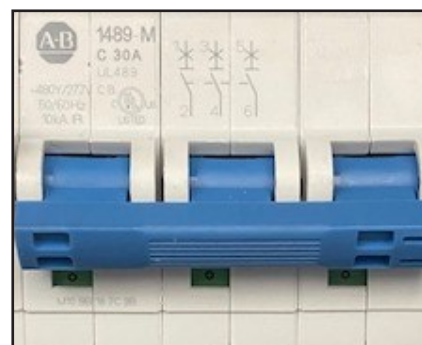
Bank 1 Breaker Open/Tripped
