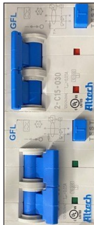
Bank 3 Breaker Closed/Hot (ON)
