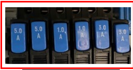
CB Bank 2 24V DC Circuit Breakers
