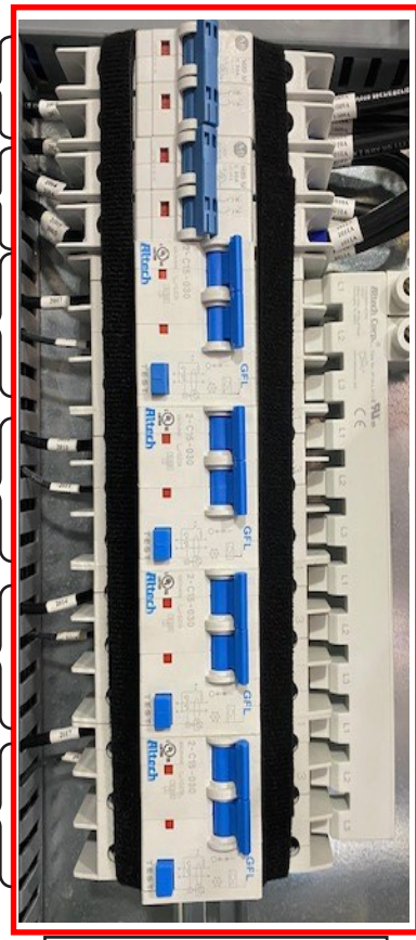
CB Bank 3 Heater Zone Breakers
