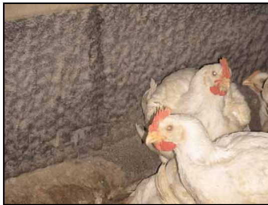
Figure 7. Very little bird damage to 10 lb/ft 3 polystyrene insulation applied to concrete stem wall.
