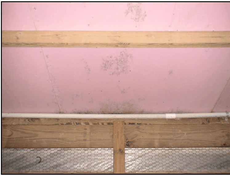
Figure 13. Beetle damage of polystyrene insulation. Dark spots are holes where beetles have burrowed into the insulation.
