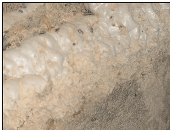
Figure 10. Bird and beetle damage where the crack between the concrete stem wall and plate was sealed using 2 lb/ft 3 foam.
